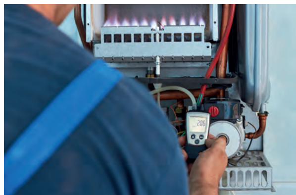
Flue gas testing on a boiler
